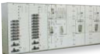
Low voltage switchgear SEV/SEK
